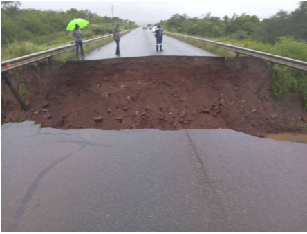
Figure 2: The washed away bridge.
